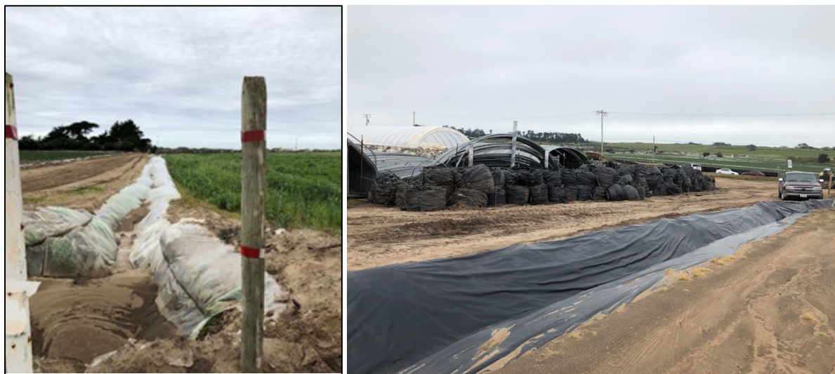
Figure 10: Plastic lined ditches control erosion but are vulnerable to breakage. Broken pieces can be transported to the ocean with storm water.
